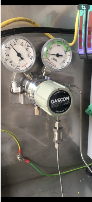
CO2 Check Valve Normal Position
