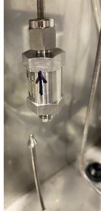
Position to Verify it Is Working Properly
